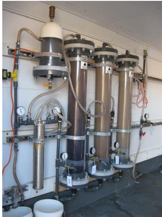
Figure 4. 3-column anion exchange pilot system
