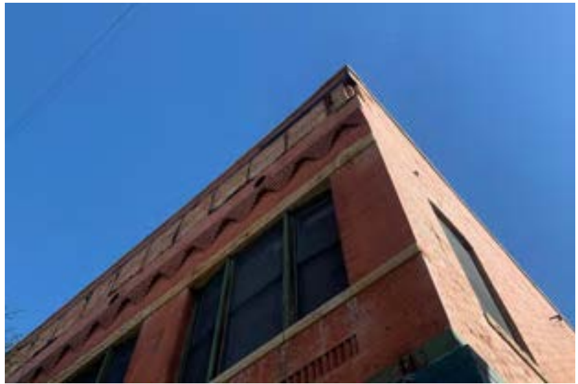
Figure 72. Coronado Building, 900-920 9th Avenue (5WL.2284). Detail of stone belt courses forming sills and lintels of upper story windows.
