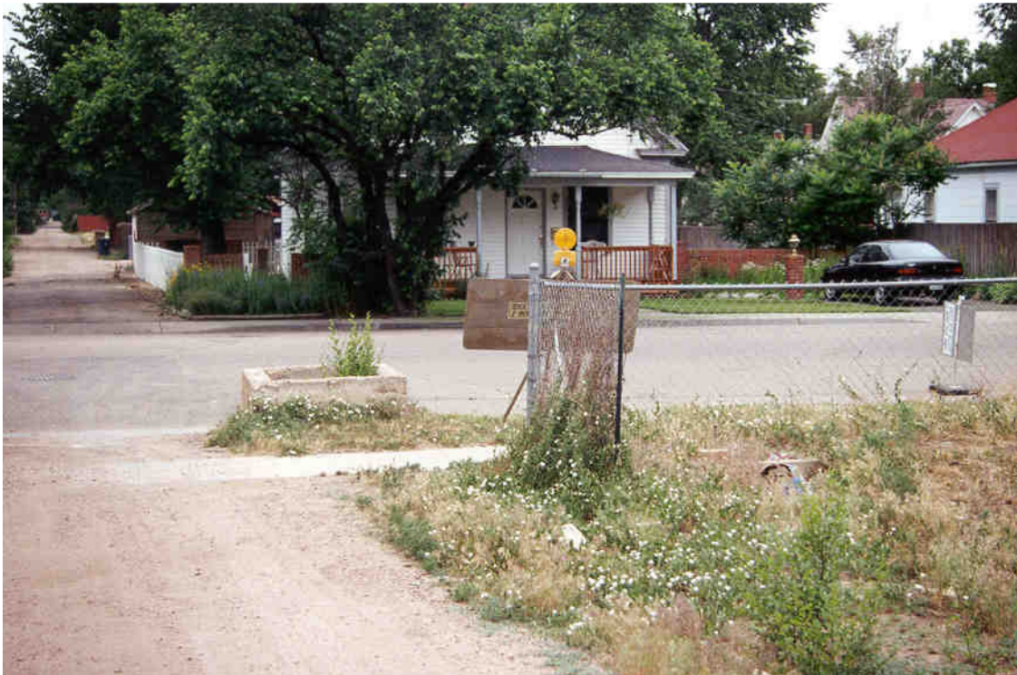
Greeley # 3 Municipal Distribution Box
