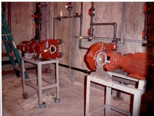
Caustic Metering Pumps at the Water Pollution Control Facility
