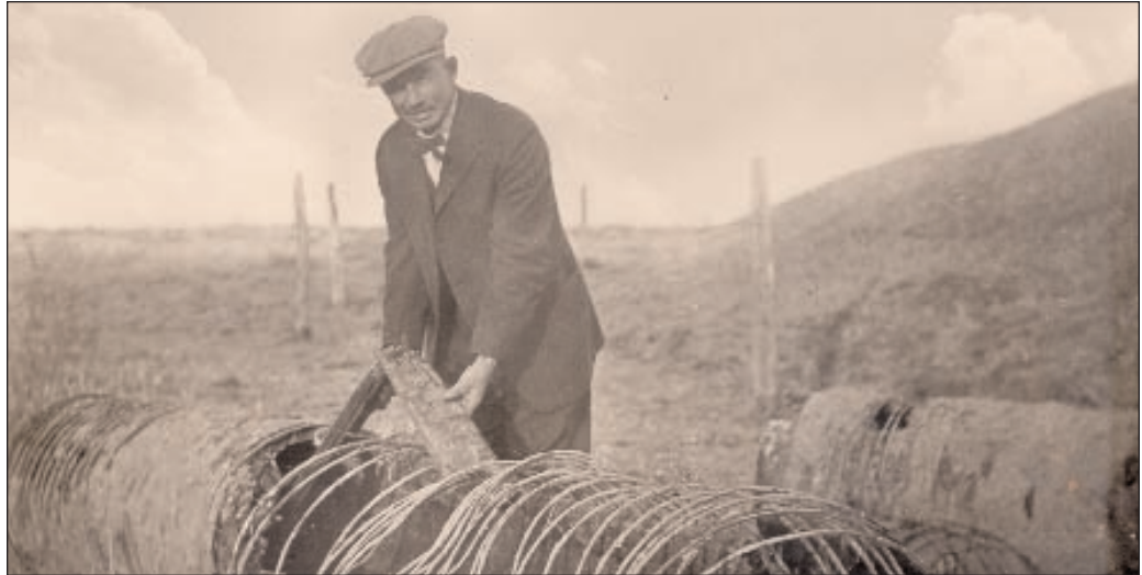
Replacing an Early Wood Water Main Source: City of Greeley Museums Hazel E. Johnson Collection
