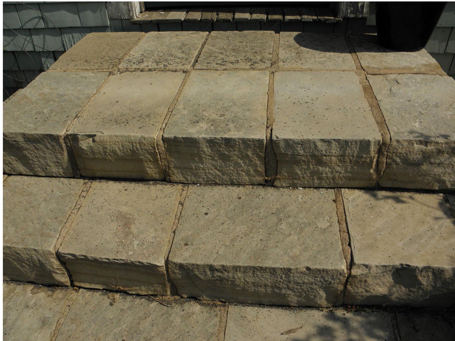
South Side – Stairs (showing gravel from the roof shingles)
