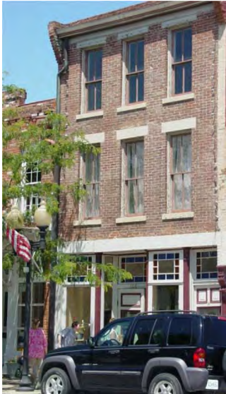
1840's Main Street building with deteriorated brick & failed caulking
