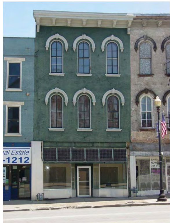
Building in the same block with original 150 year old windows & wooden storms.
