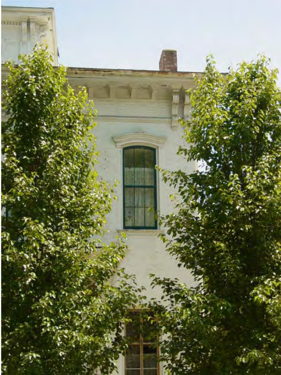
1859, six over six, true divided light historic window with a wood storm. The storm does not obstruct the view of the window
