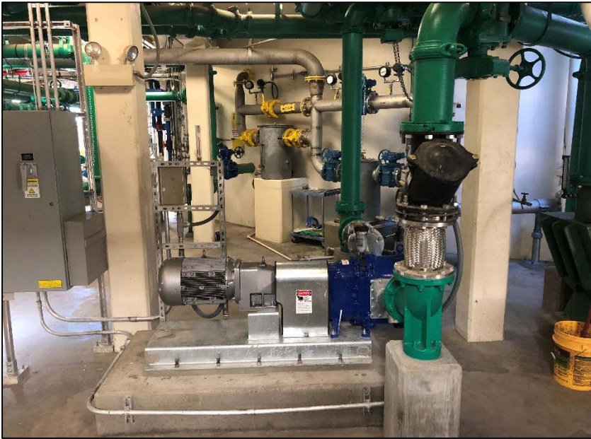
New sludge transfer pump inside digester building.
