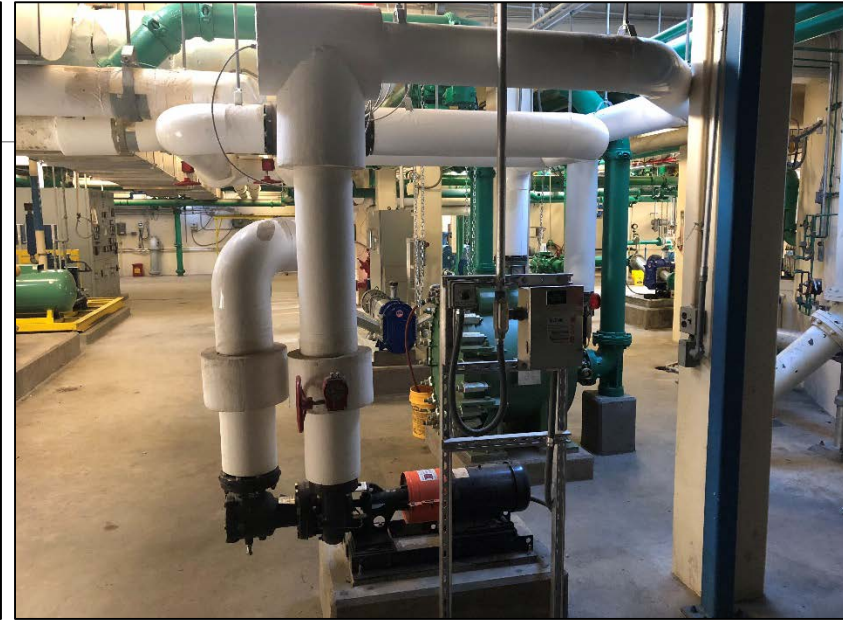
New sludge piping inside digester building.
