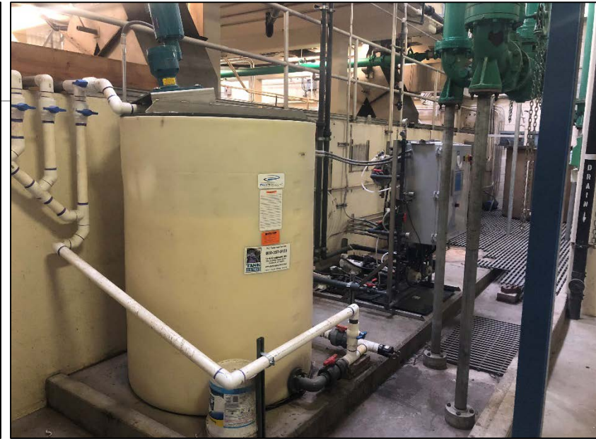
New polymer mixing equipment inside digester building.
