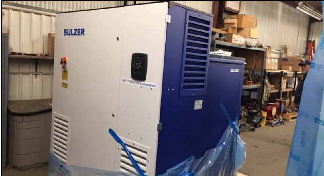
New Sulzer Blower Units
